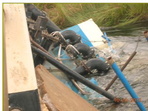
Water pumping station in Soroti damaged and overrun by flood waters
